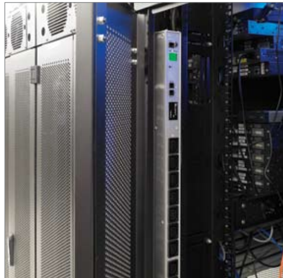
Figure 4. Racks with vertically mounted intelligent power strips.
