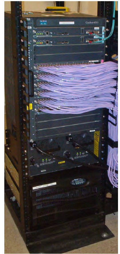
A network closet at Marquette.
